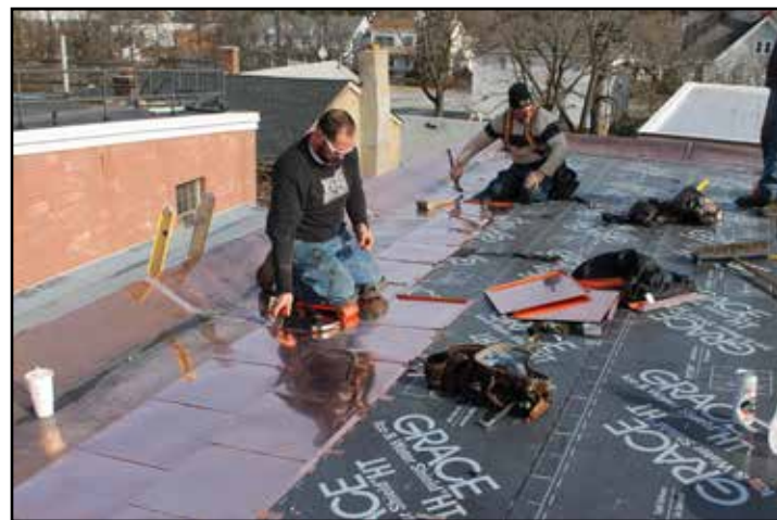
The crew installs interlocking copper pans above the continuous gutter. To finish, all seams will be soldered.
