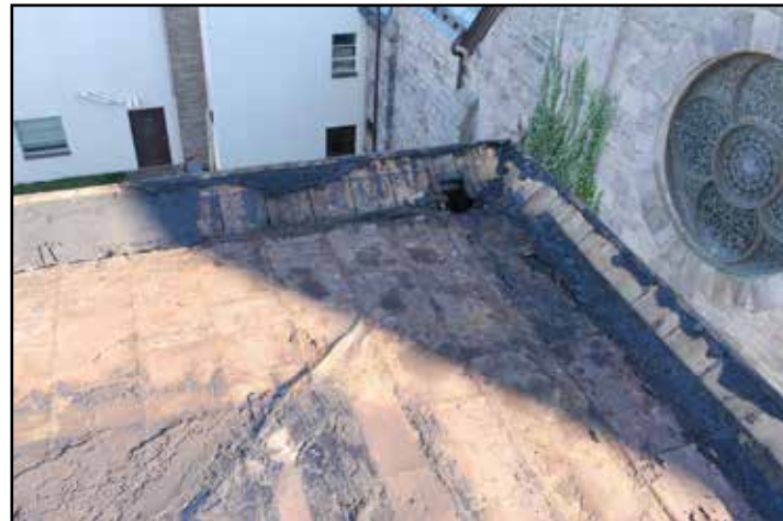
Original materials uncovered after 170 years: rusty sections of tin roofing and pine gutter-sheathing boards.
